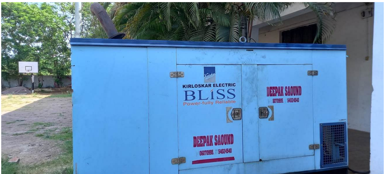
DG set of 82.5 KVA rating
